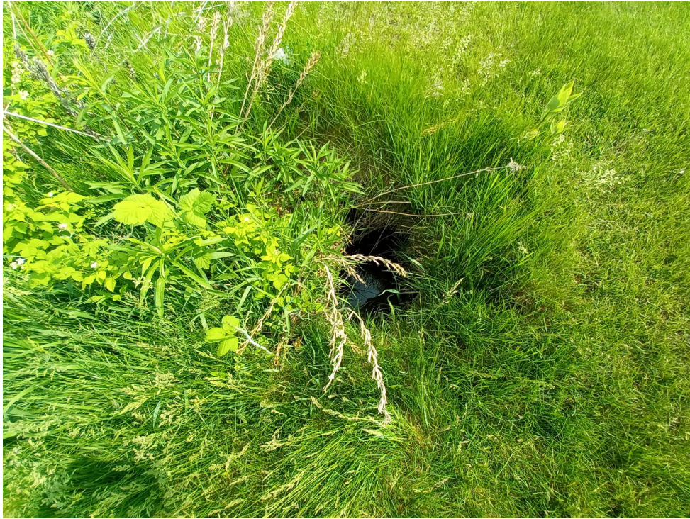
Photo #4: Sinkhole at southeast corner of basin. Appears to be caused by a joint separation in a storm sewer pipe meant to discharge into the basin. This is on the neighboring property at 1420 Stamy Road.
