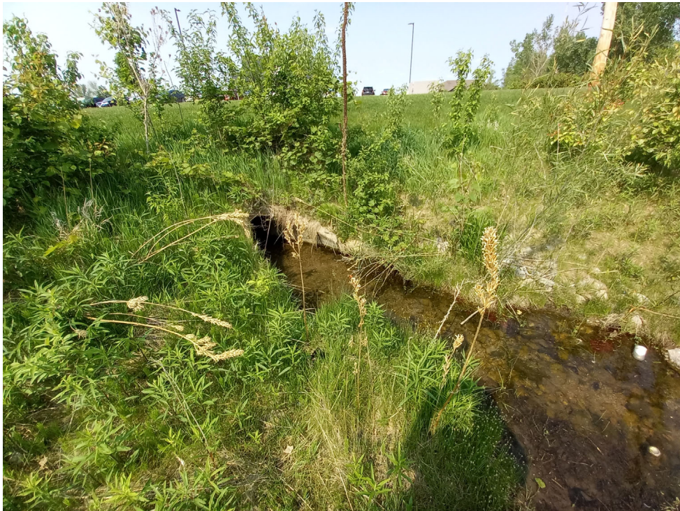
Photo #7: View of the storm sewer pipe discharging into the southwest corner of the detention basin.
