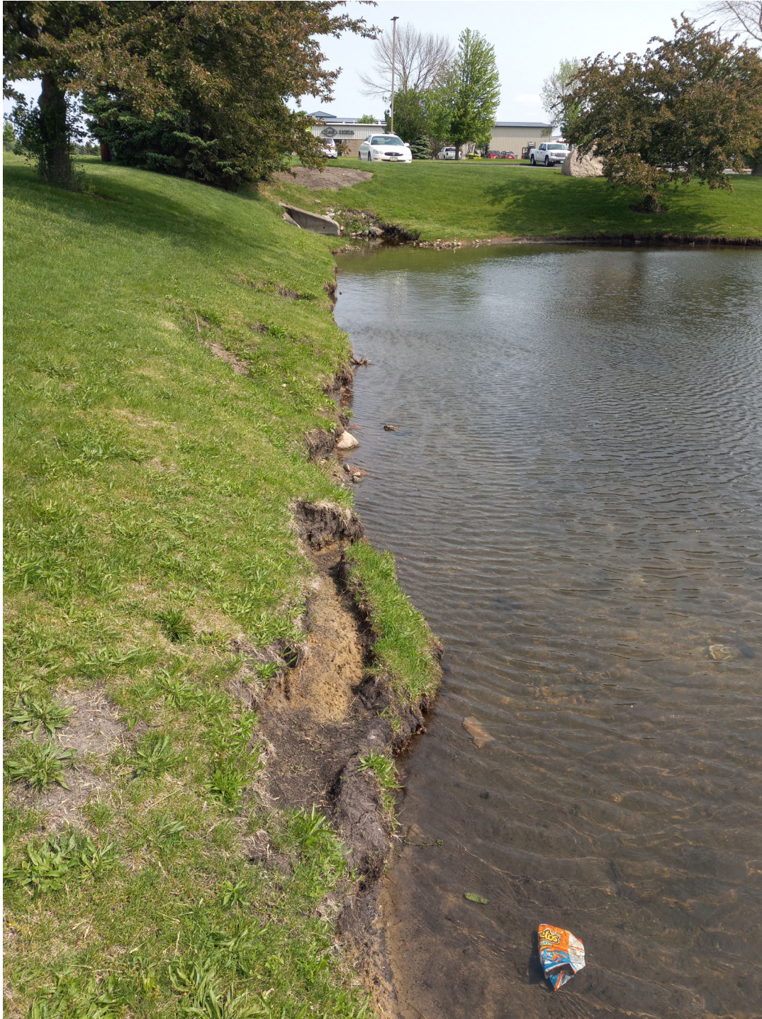
Photo #10: View along the basin's west bank, north of outlet, showing bank line erosion and sloughing.
