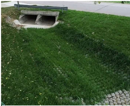
Northwood Drive Detention Basin
