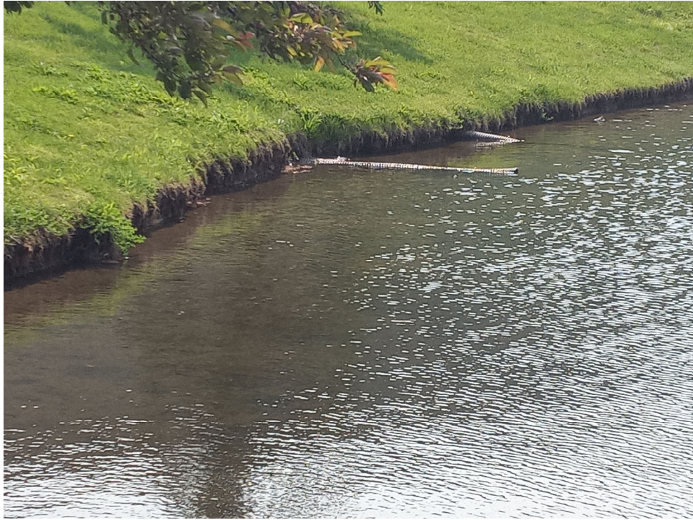
Photo #11: View along the basin's east bank, showing bank line erosion.
