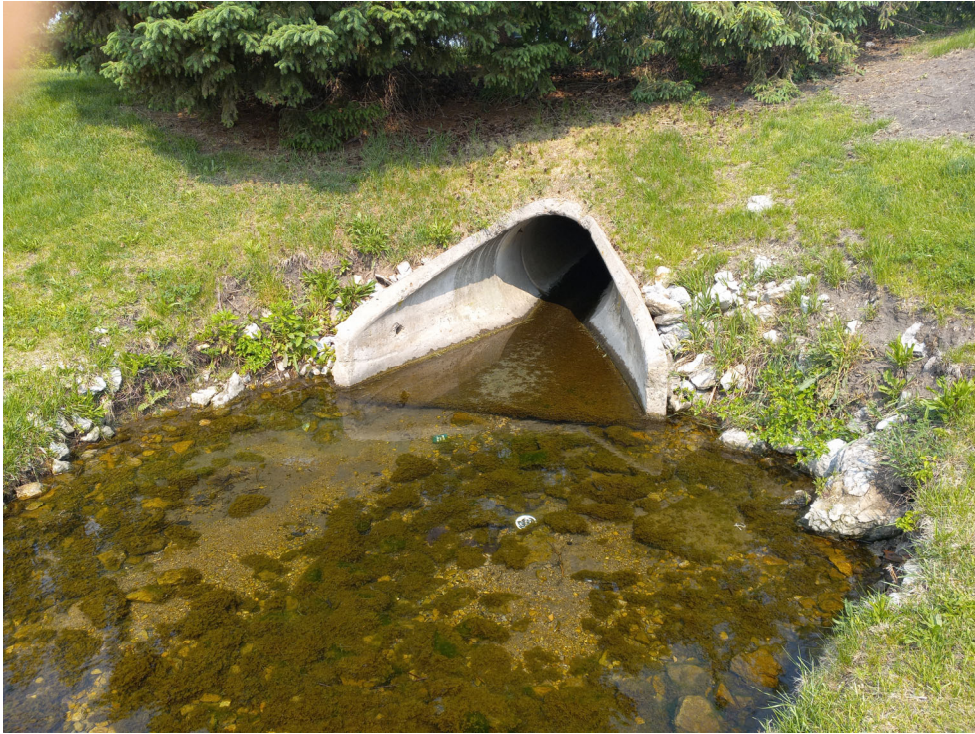
Photo #2: View of the storm sewer pipe discharging into the northwest corner of the detention basin.
