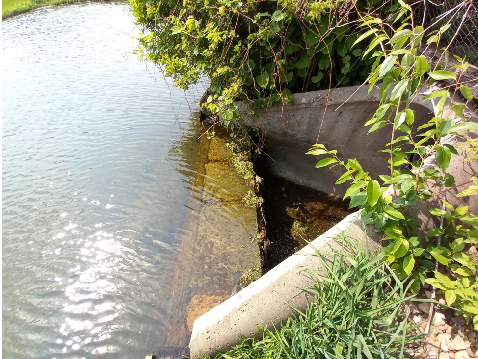
Photo #8: View of the detention basin's outlet, which is a 54" diameter concrete storm sewer pipe with a flared end section and an approximate 24" high concrete weir across the end of the flared end section.
