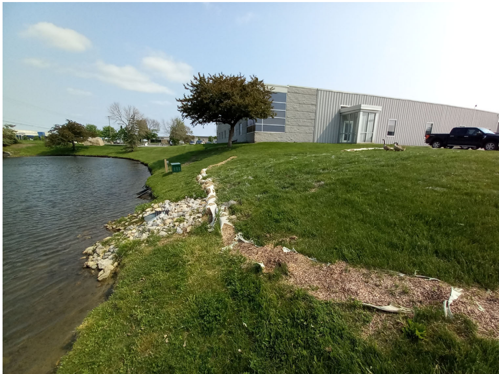
Photo #3: View of the storm sewer pipes discharging into the east side of the basin. The outlet with new rip-rap was recently installed with the parking lot addition for the subject property. The section of the bank that was disturbed for the storm sewer installation is nicely vegetated and restored. The filter socks installed served their purpose and are suitably degrading and becoming part of the landscape.
