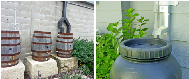
Left: Connected rain barrels capture more water for reuse. Right: A downspout is redirected into a rain barrel.
